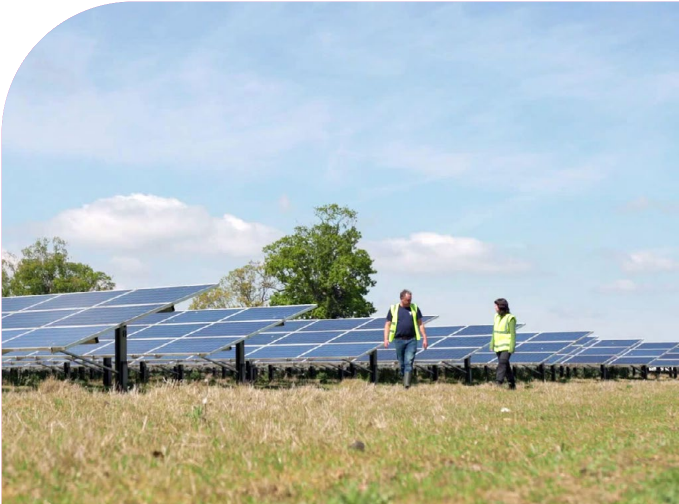
Honington Solar Asset (UK), NextEnergy Solar Fund
